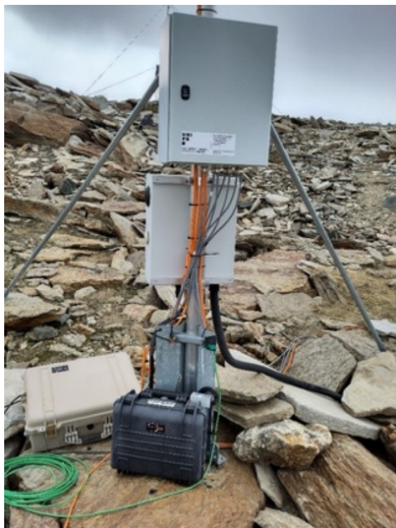
Figure 4.1. Electrical Resistivity Tomography (ERT) monitoring installation at Stockhorn. Photo: C. Hilbich.
